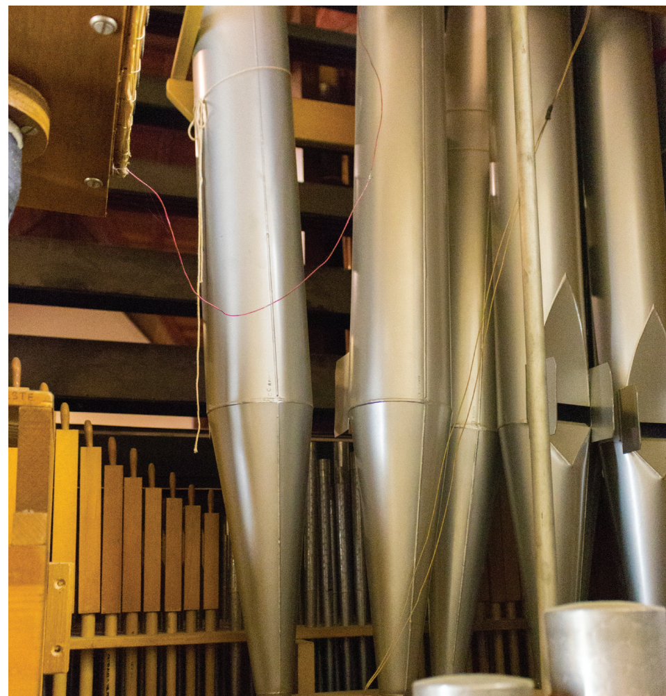
View of the “Mish-Mash” of crowded pipes in the existing main organ chamber.
